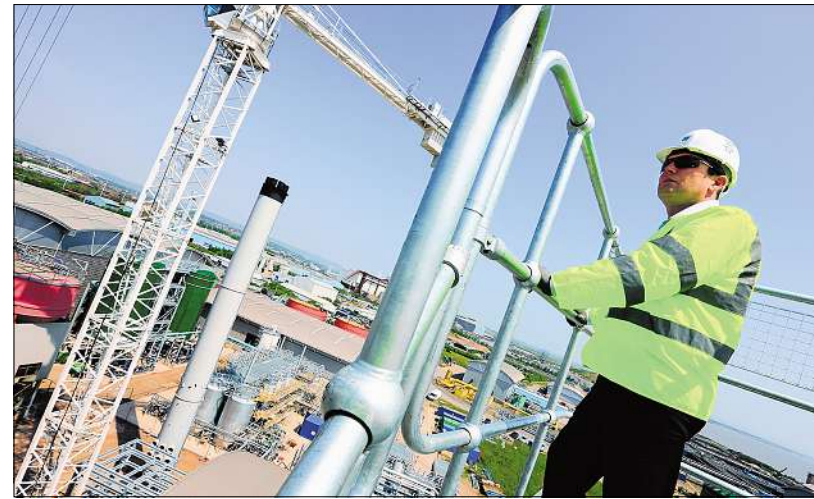
In the past five years the company has spent £1.4bn on improving drinking water and sewerage systems
