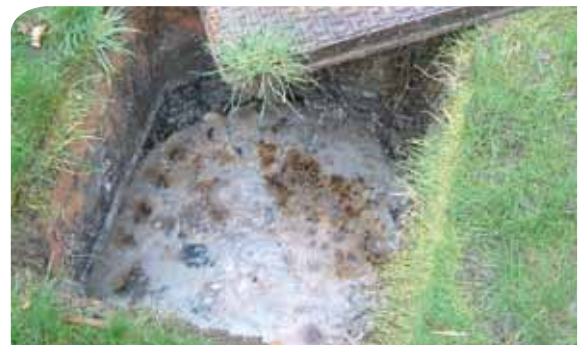
Fat building up in a manhole Braster mewn twll archwilio
