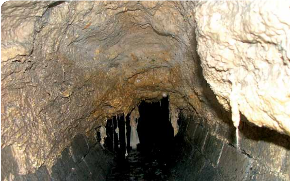
Fat beginning to block a sewer
